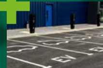
Fast car charging (EV)
